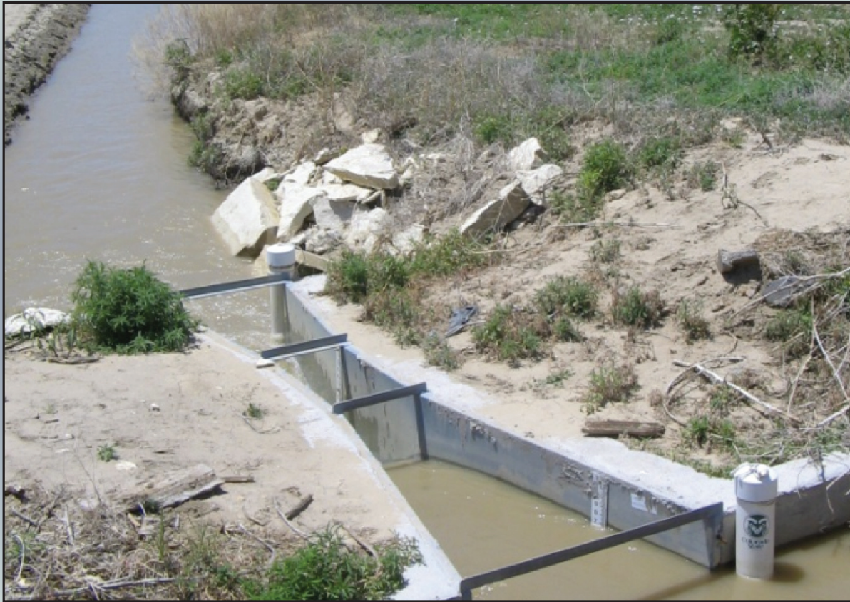
Figure 13. Permanent measurement structure for inflow to Field DS6, provided by Fort Lyon Canal Company during seasons 2005-2008
