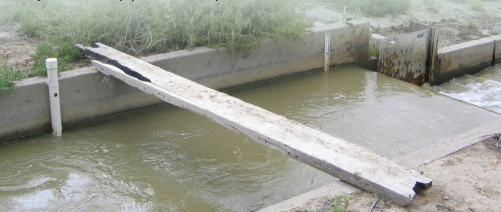
Figure 14. Weir structure for flow measurement onto fields DS4 and DS16 in 2008
