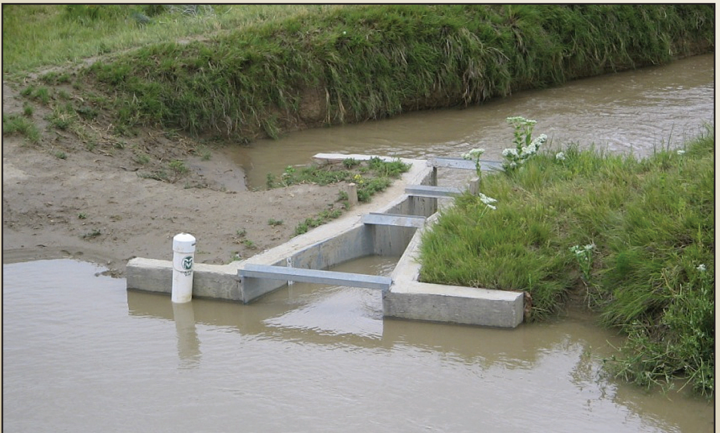
Figure 16. Parshall flume for measurement of flow to field DS1 in 2008
